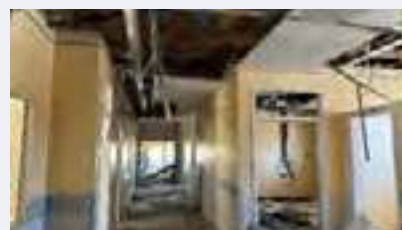
Facility after vandalism
